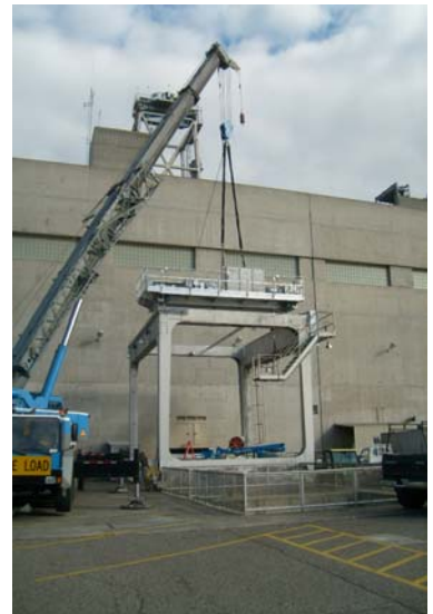
ACT sets the new 50/5 ton trolley on the tailrace gantry crane at Lower Monumental Dam, Snake River, WA
