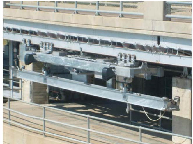
10 Ton Spillway Crane—Gavins Point Dam, South Dakota
